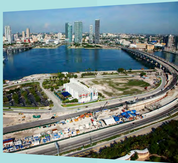
Port of Miami Project in Florida, U.S. 250,000 cubic yards of ready-mix concrete
