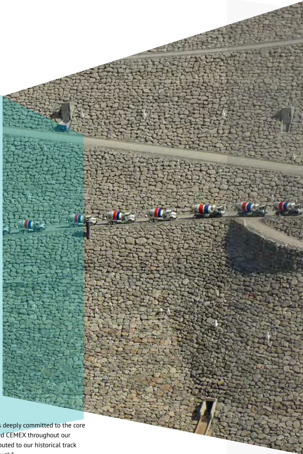
La Yesca Dam in Jalisco and Nayarit, Mexico Two dedicated ready-mix concrete plants installed for construction of the 207-meter wall
